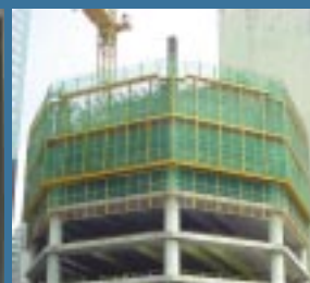
External reusable floor edge protection fencing
