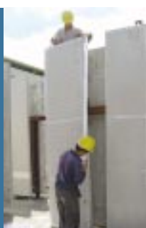
Lost formwork wall panels
