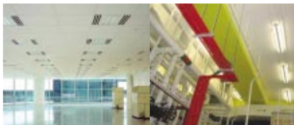
T5 fluorescent tubes installed at Cambridge House
