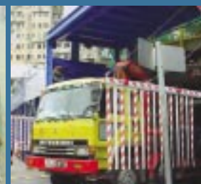
Safety barrier for pedestrian flow control at site entrance
