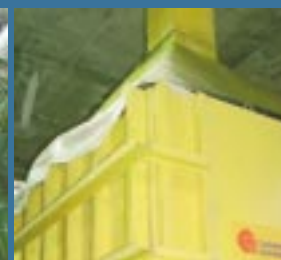
Dust suppression chamber at Three Pacific Place
