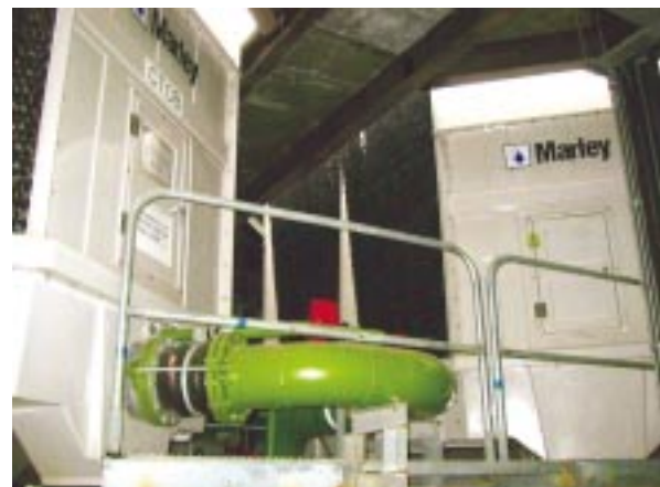
Water cooling towers
