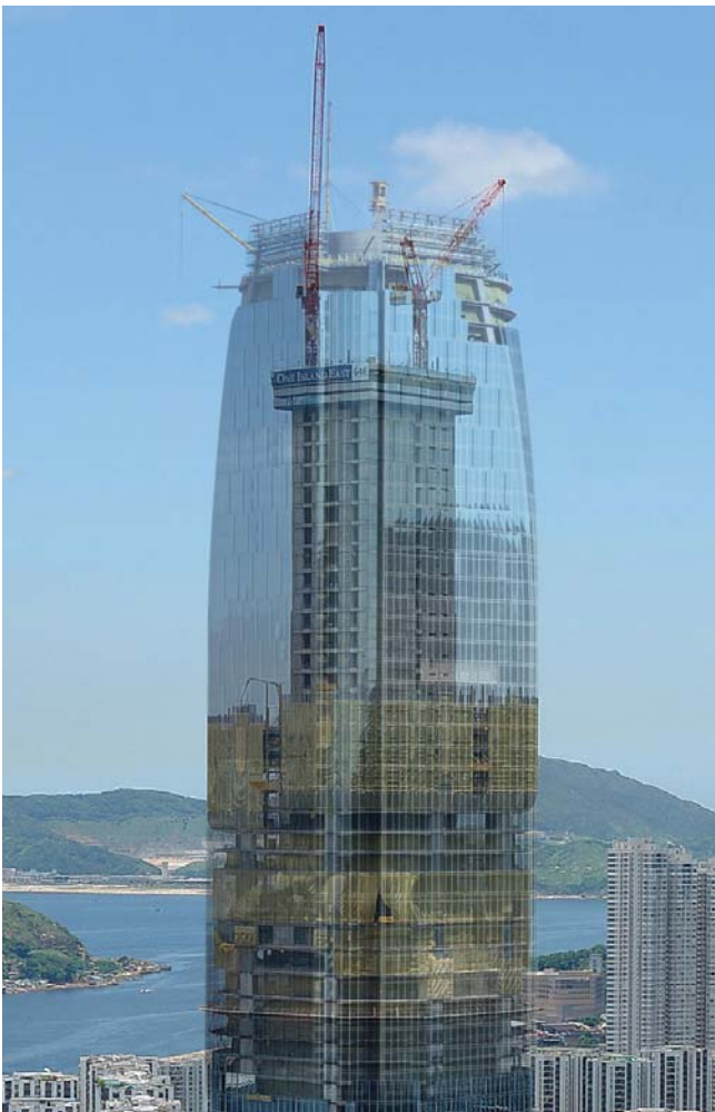
Building Information Modelling was used during the construction of One Island East
